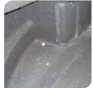
Examples shown are of unacceptable damage.
